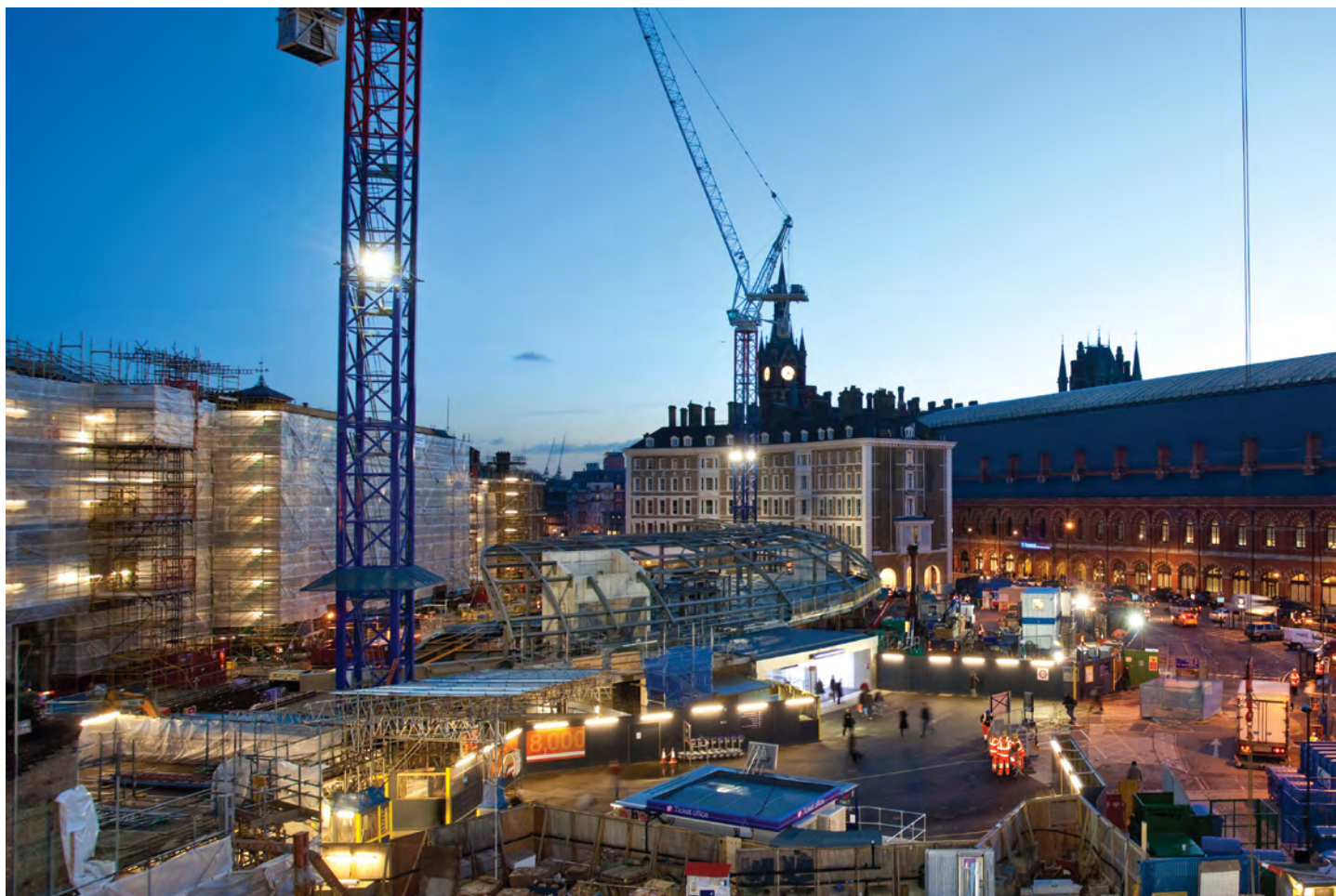
Construction activity for the new King's Cross Station's western concourse and the Great Northern Hotel in the background
