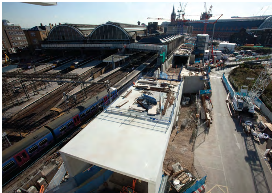
The Shared Service Yard will be accessed from Goods Way via a ramp down to basement level
