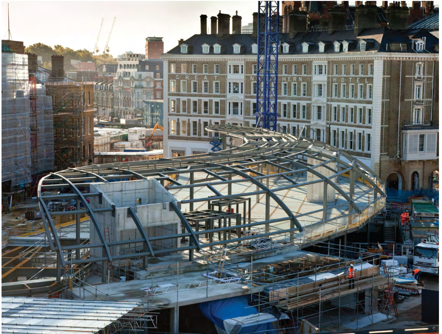
Network Rail's new concourse for King's Cross Station, being constructed by Taylor Woodrow, with the restored concave façade, by Kier Group of the Great Northern Hotel in the background
