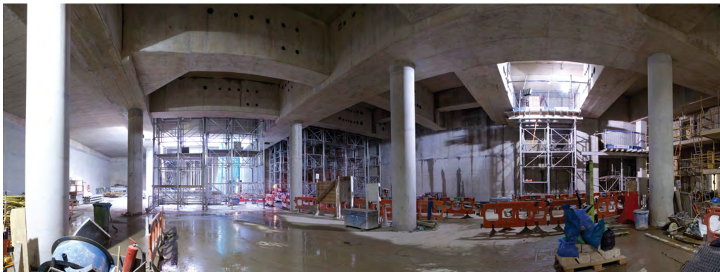
Double height Shared Service Yard allowing vehicles to off-load goods and service offices and the station above
